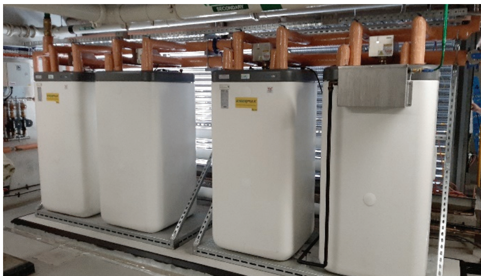
The highly insulated thermal storage tank reduces energy waste from heat loss.
