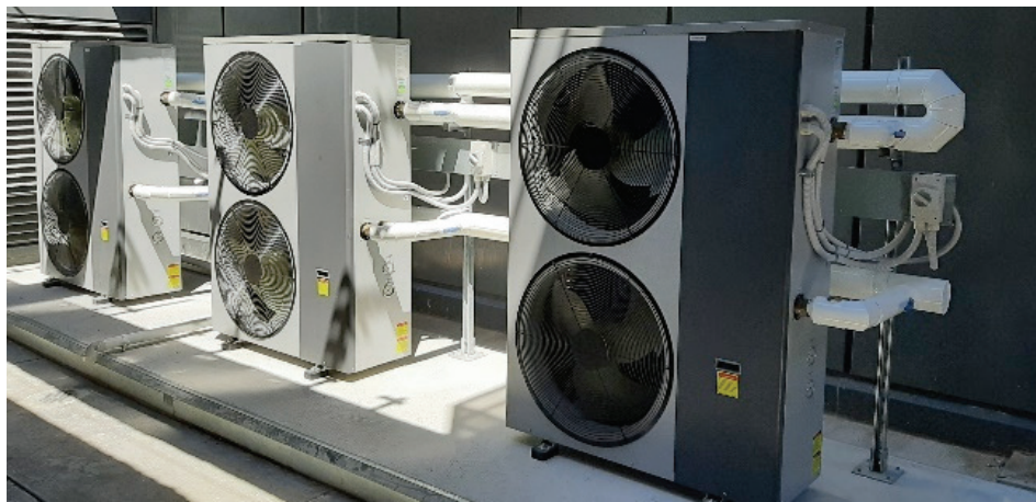
The heat pump units.
