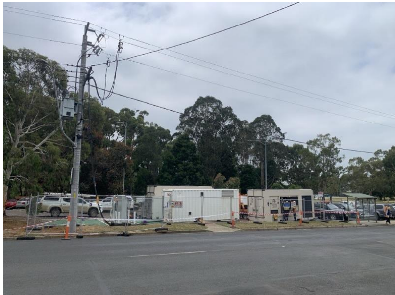
Figure 21: Picture showing large generator and temporary connection to local electricity grid.
