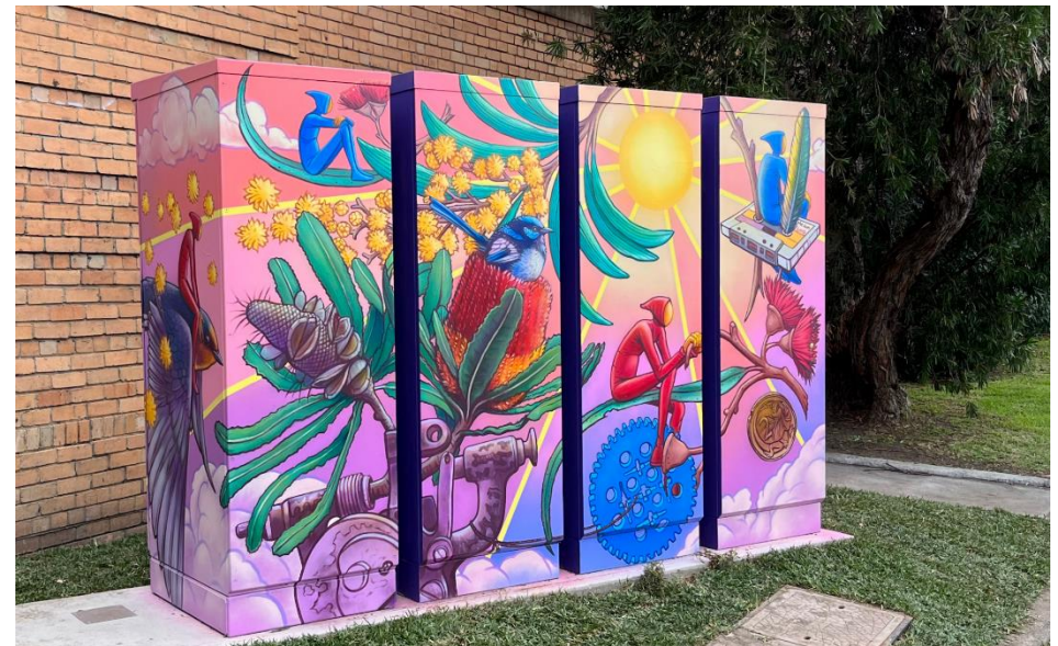
Figure 1: YEF's Fitzroy North Community Battery (FN1), delivered in 2022 with funding from the NBI
